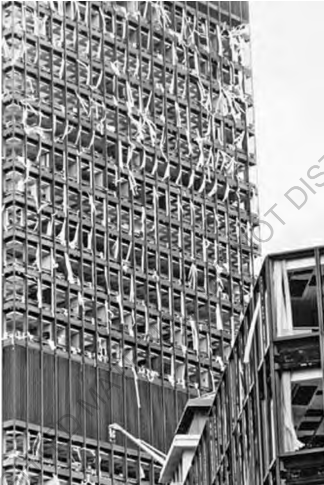
Figure 2.6 Widespread blast damage to conventional glazing
