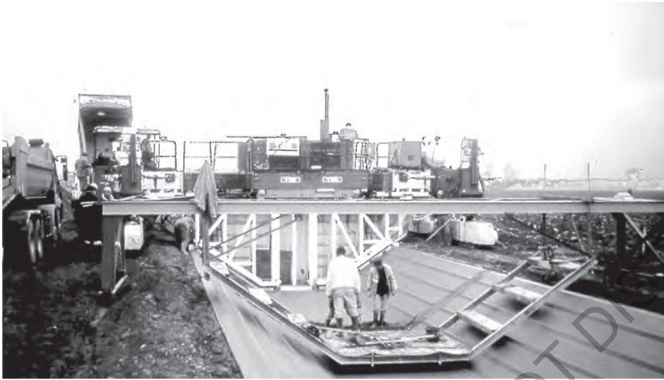
Figure 16.9 The Mulhouse Canal (France) – extruded concrete sliding formwork machine. (Courtesy of D. Croissant, Cemagref (1997))
